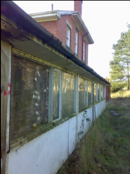
ABOVE & RIGHT: Hmm. There's an awful lot of these covered walkways about, on both sides of the spikey fences, but how to get into them? Luckily, hardboard is not known particularly well for its weatherproof properties and in a few places wasn't particularly weatherproof or well attached at all, which was to our advantage.
