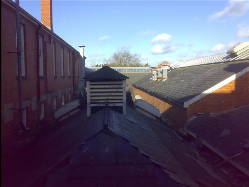
ABOVE: Chim chimeny, chim chimeny etc. is that a much denuded and rusting exposed roof support we can see just to the top right of the skylight? That would be the hall then.
