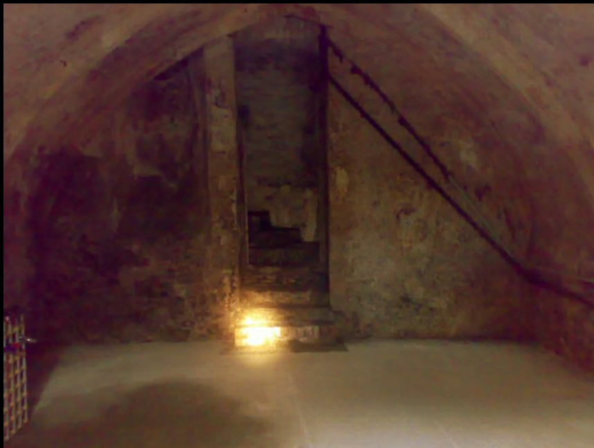
BELOW: Detail shot of the back staircase up to the room above, or possibly the courtyard. In this instant it's been boarded over and probably made into another small room above: a bit of a shame as it would have been an incredible feature to retain.
