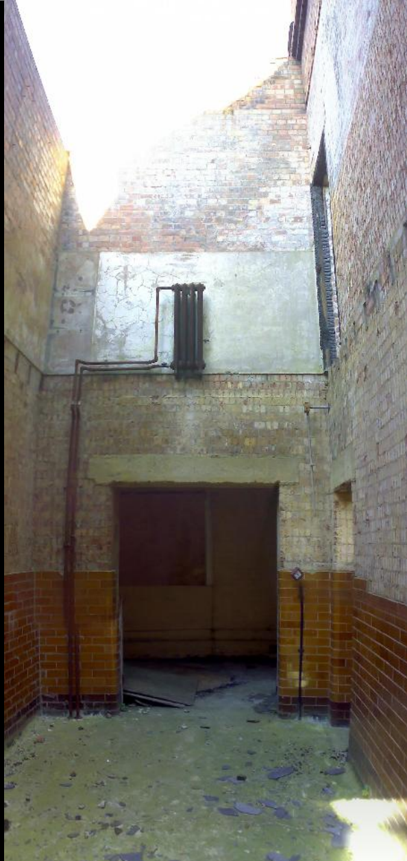
ABOVE: What we would consider to be a challenging plumbing job. Obviously, there would have been another floor overhead and despite no evidence of burnt roof members in this area on the floor, the joist holes in the walls and changes in rendering support this hypothesis.
