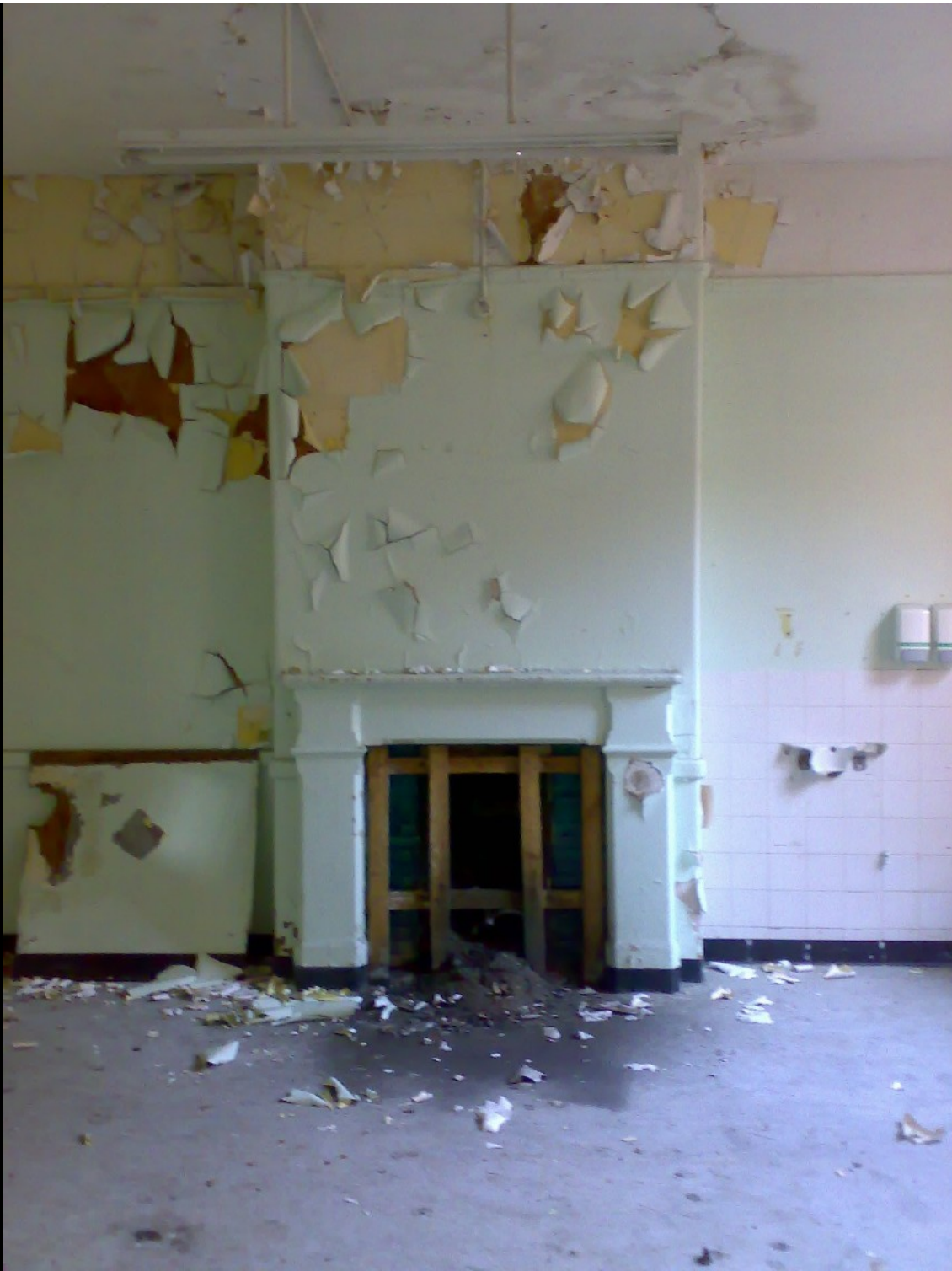
ABOVE: There were some pretty fireplaces in this area, all boarded up and forgotten about. I personally really enjoy a nice open fire, but I can see the disadvantages of having them in a building full of lunatics...
