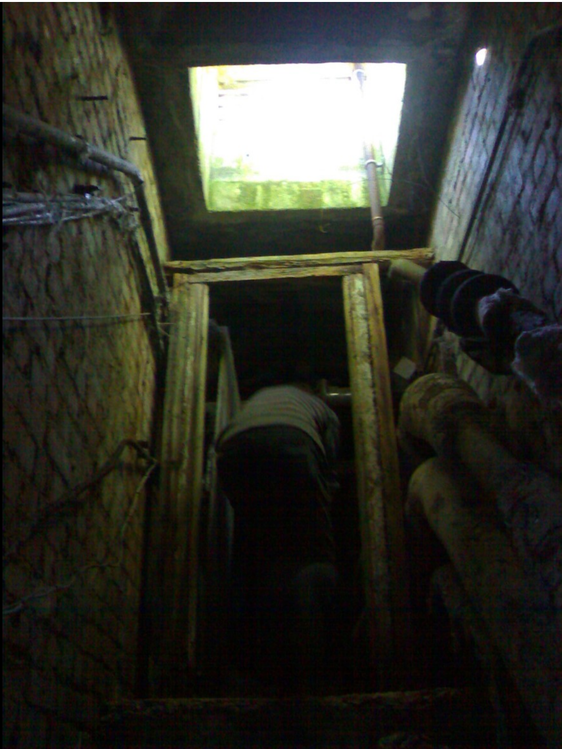
ABOVE & BELOW: We couldn't leave the place without a quick blast in the service tunnels. Sadly, whilst we had brought a torch with us, Agent Skyframe had left it in the car, so we spent most of our time in the tunnels navigating by the light of 2 mobile phone screens, which was intense to say the least. As a result, we didn't really get any amazing photos from in the tunnels, but we did end up under the little hatch that we had found on the way in! It was very weird seeing it from the opposite way round and took us a little while to get our bearings.
