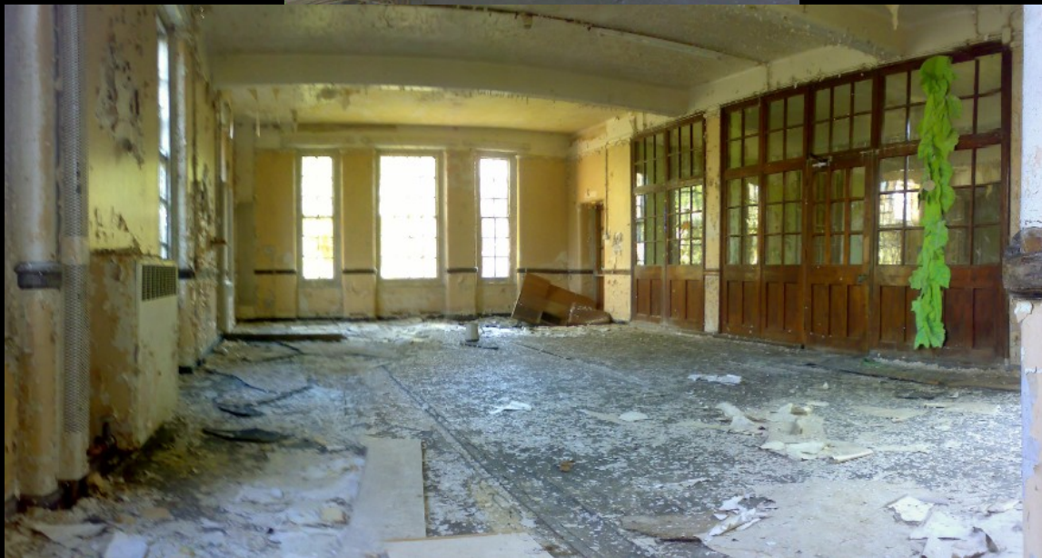
ABOVE: After a good look around the Occupational Therapy Department, we returned to the ground floor in order to move on. The hole in the floor we used to gain access is on the right, just out of shot.
