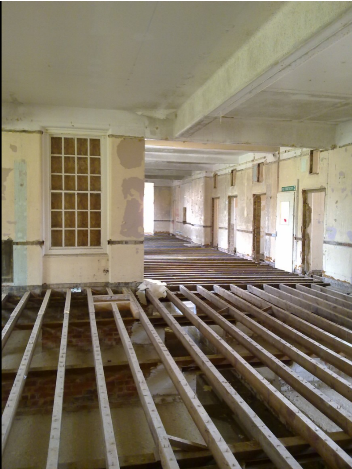
BELOW: In some places, the door frames, picture rails and wooden valance strips had been removed and we wondered as to the reasons they had been removed so carefully. Maybe the intention was to put them back or render over the doorway here, but usually, blocking up of a doorway would be a lot rougher, due to the need for edges to key new brickwork onto. Again, the ceilings have been very carefully and tidily removed, giving us hope that this place will be reused.
