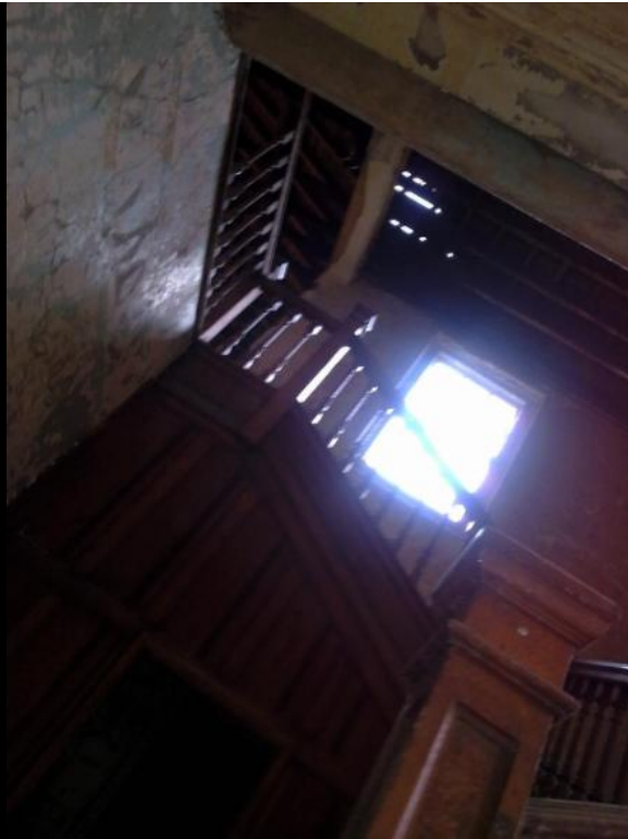
BELOW: More stripping out. This location doesn't look to be in fantastic condition, so is probably for the chop. Very sad.
