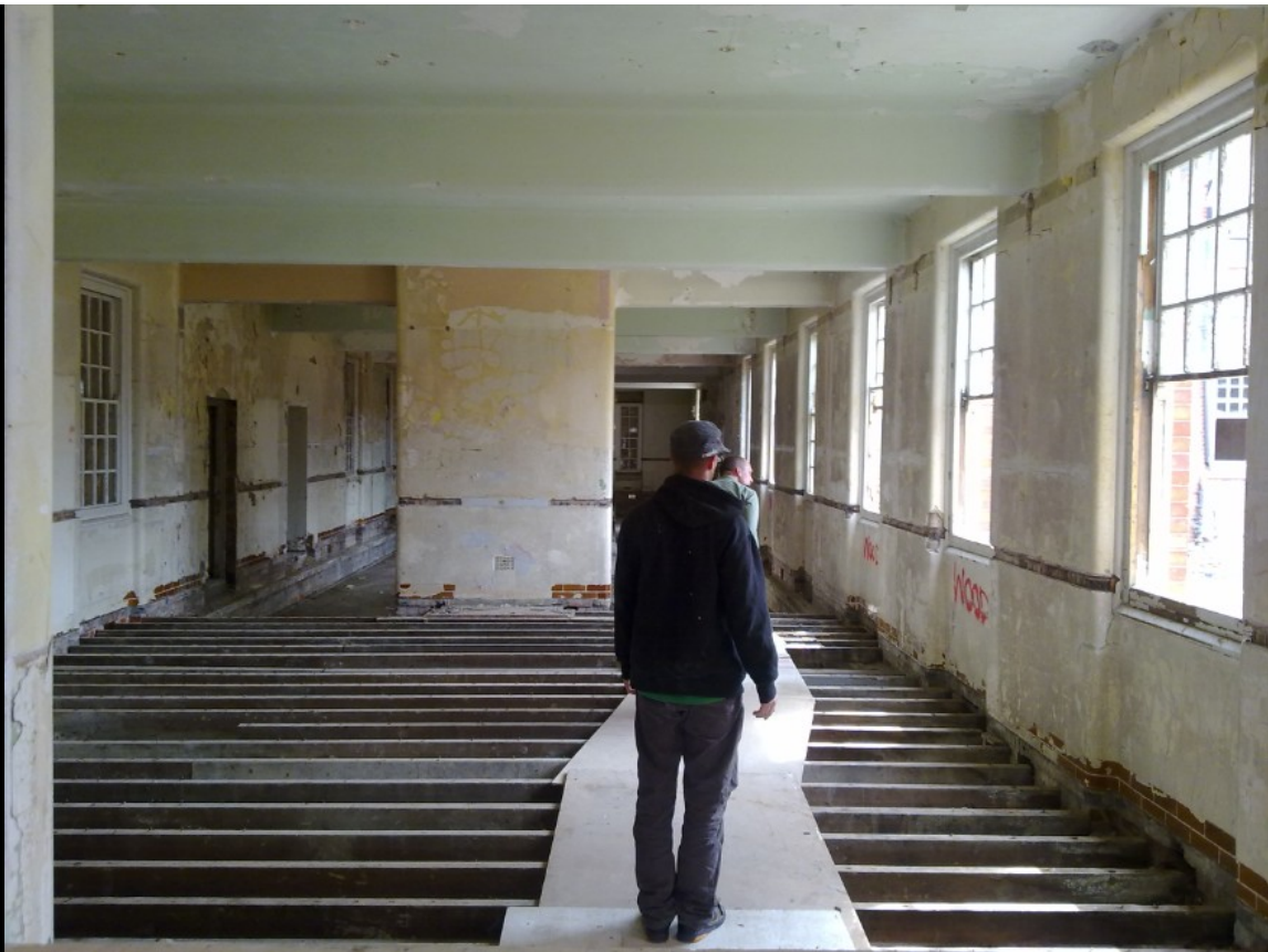
BELOW: In the next room along, we became increasingly thankful for the impromptu walkway, as the drop into the underfloor void deepened considerably.
