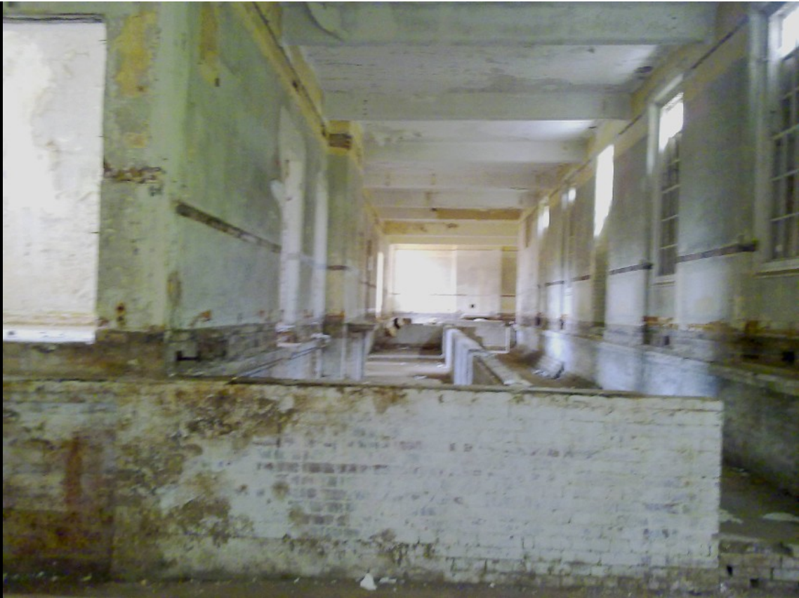
ABOVE & BELOW: floorboards had been removed, leaving an interesting maze of little walls that would have made up the underfloor void. None of the brickwork had been removed as yet, so this gave us hope that maybe this location would be saved and converted; the structure appeared to be sound in this Villa and very much more so than in some of the more popular locations we had seen before. There was no water damage and the internal paintwork and render looked very sound.
