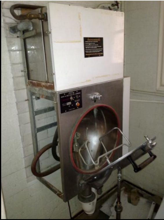
ABOVE: Unnecessarily complicated bedpan washer.
