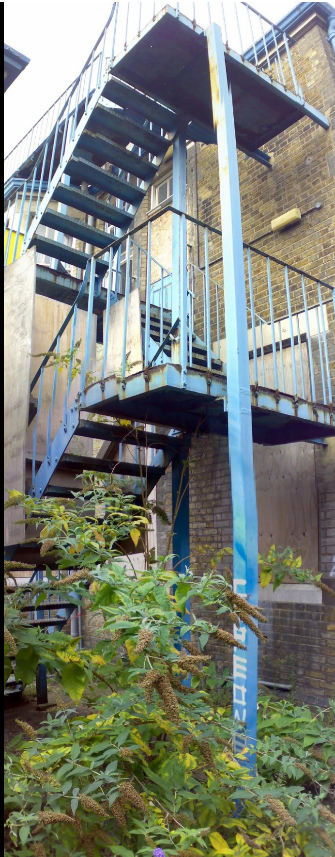
BELOW: This stairwell opposite the fire escape looked curious, but was locked and screwed shut! Damn damn damn!!
