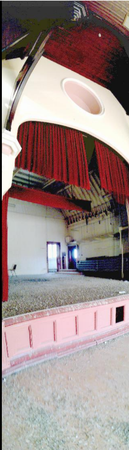
TOP RIGHT, CLOCKWISE TO TOP LEFT: The upstairs hall, detail of the stage, complete with quite a nice lighting rig and several tonnes of pigeon poo, the flies and more fantastic roof support detail.
