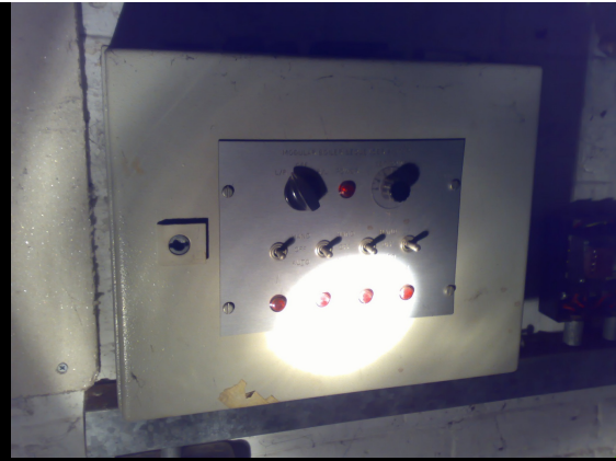
ABOVE: Live and kicking! The electrical switchgear down here was giving off a worryingly "used" sounding buzzing....
