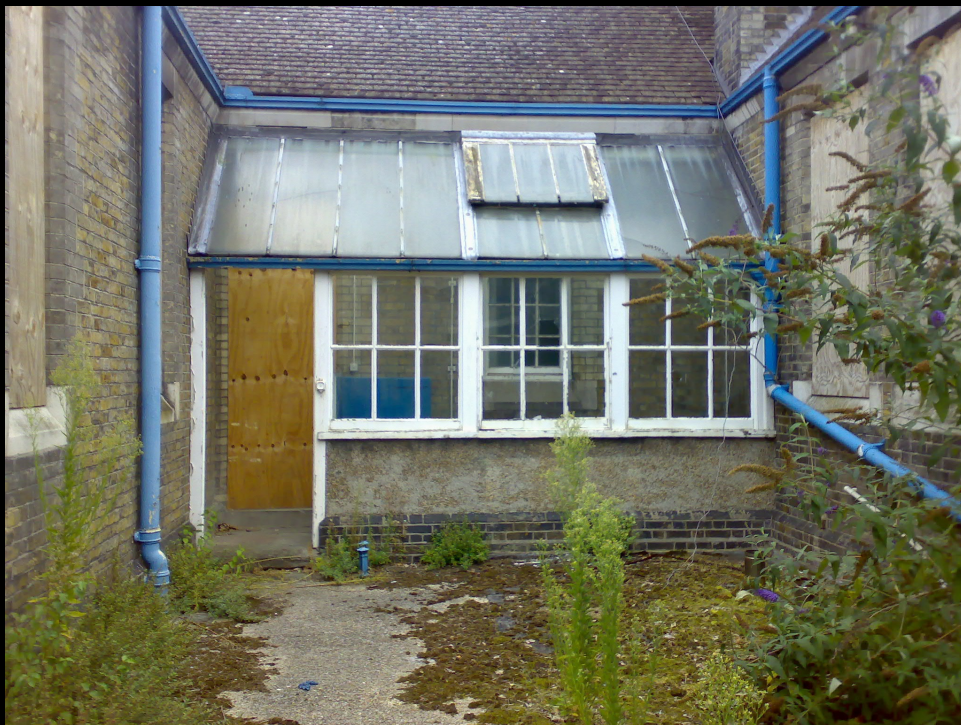
ABOVE & BELOW: The door was open and it looked quite promising. However, the window behind wouldn't open and a stairway lead down to a boiler room. Was this the sweet spot?
