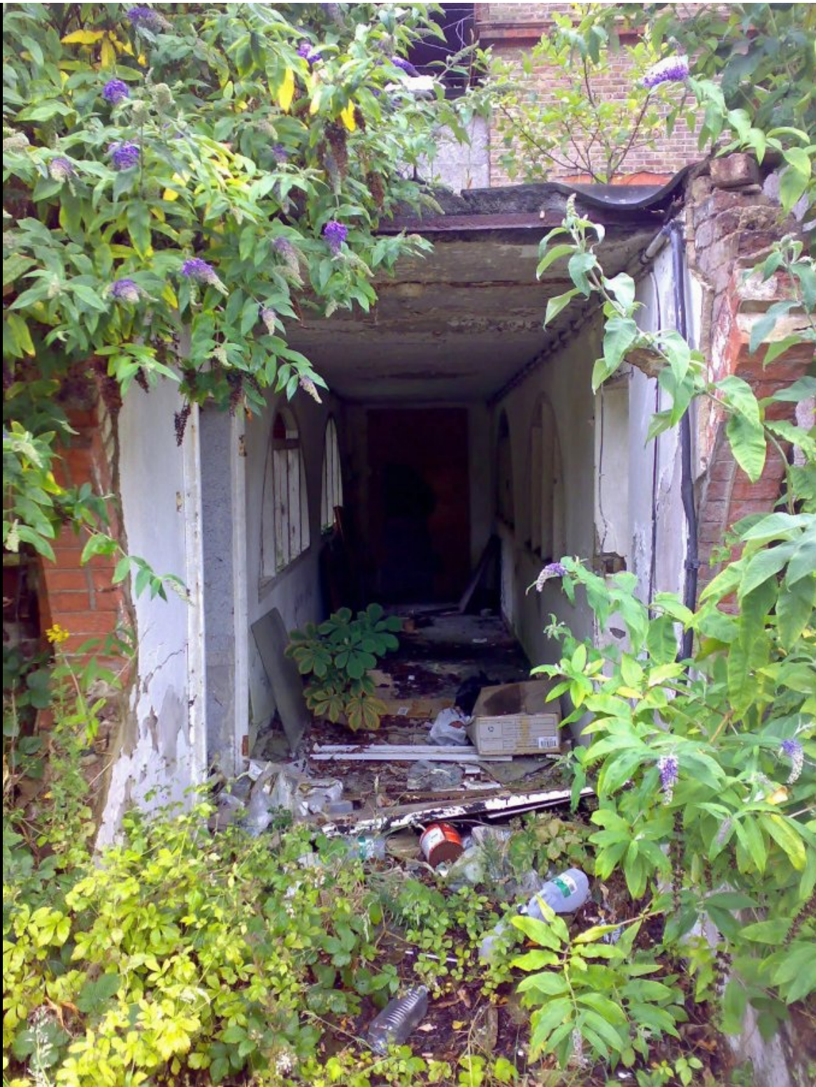
BELOW: The view to the left (east) of the walkway and the eastern end of the building. The pathway marked out by the orange webbing leads to more modern buildings to the south-eastern quarter of the site.
