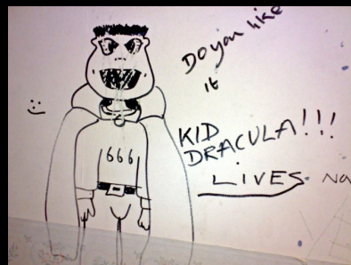
BELOW: This building has been empty and unsecured for quite some time. As a result, the vandalism was pretty bad in places.
