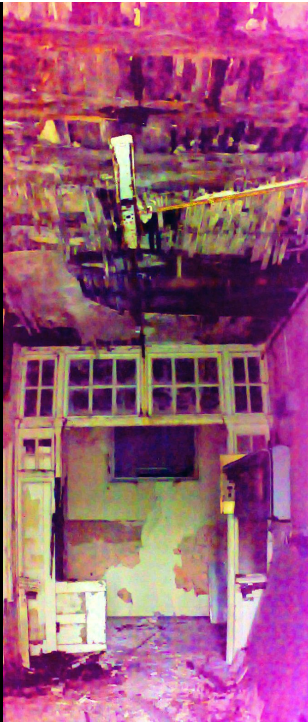
BELOW: Whilst nothing near the same scale as Hellingly and West Park, this little hall was still an interesting find - it had a lot of atmosphere (and bird shit) and must have been quite nice in its day.
