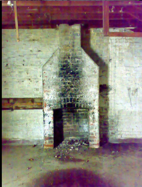
RIGHT: There was a row of what looked like stables on the western perimeter wall of the site. Some of them had these little fireplaces in. Curious. We wondered if they were forges.
