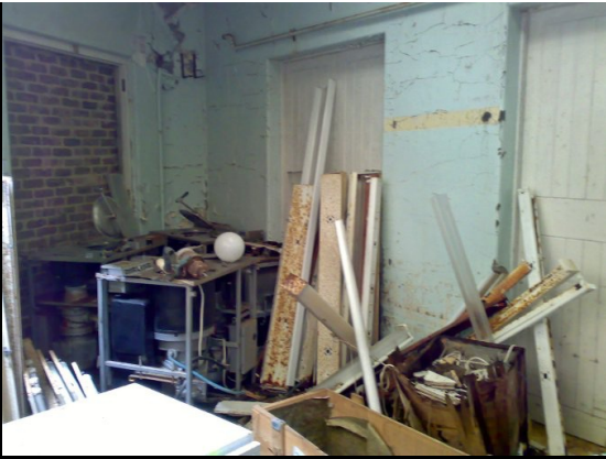
ABOVE: The first group of buildings we found were outbuildings on the northern perimeter wall and were clearly used for storage. Part of these had been assigned to an engineering discipline, the others were more general maintenance and I.T.
