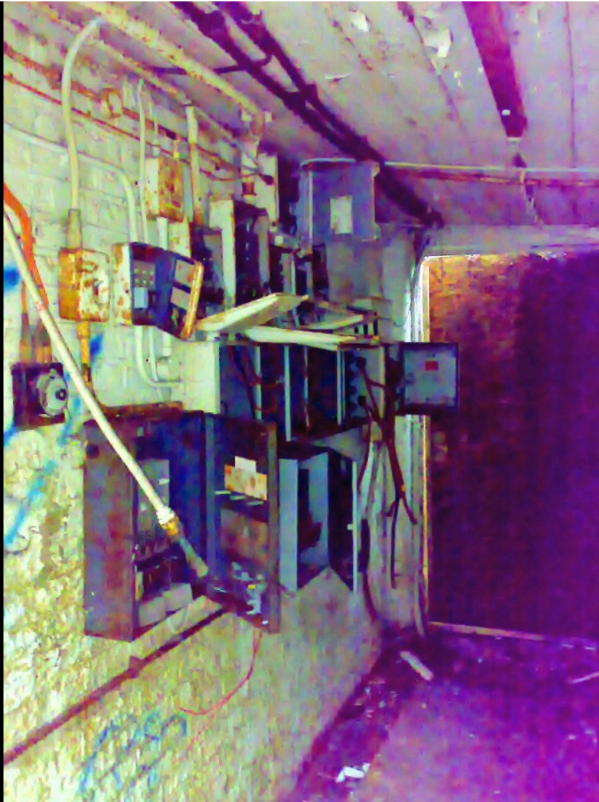
ABOVE: The majority of the electrical installations we found had been stripped out and were pretty trashed. Again, we couldn't be sure if this had been done by metal thieves previously, but this time it looked more methodical, so we are guessing that as parts of the site have been removed, they have been isolated and removed from the electrical layout gradually.
