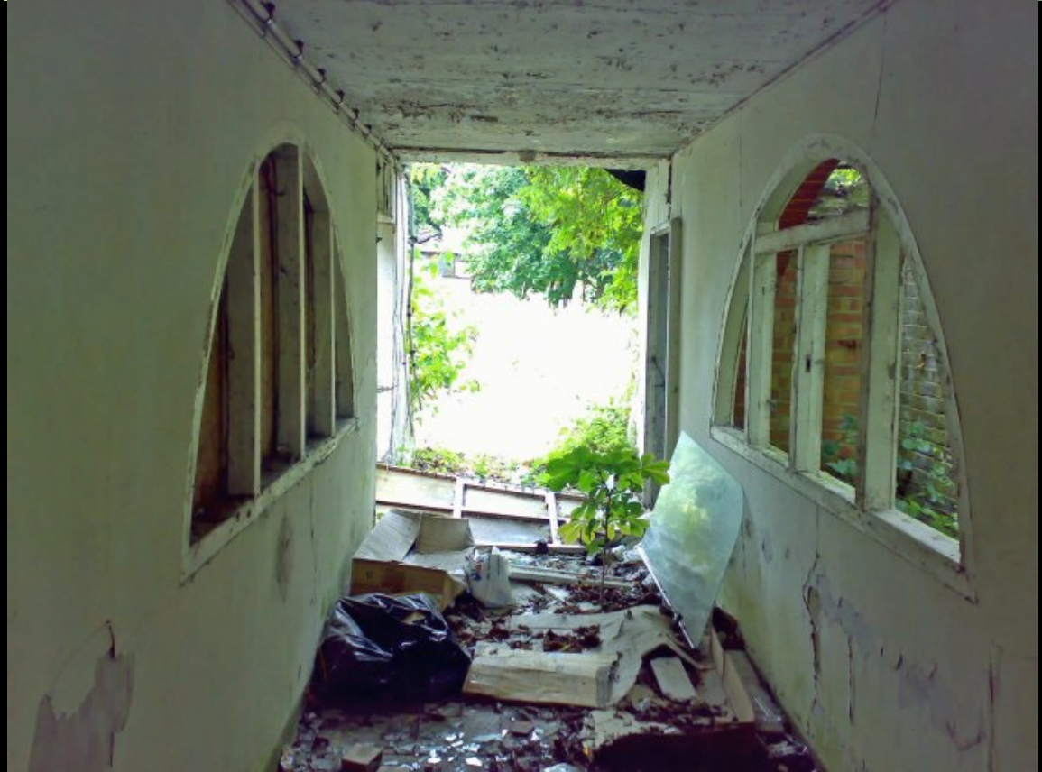
ABOVE: The corridors that remained had incredibly ornate and interesting curved windows, which must have been quite expensive to get replacement glass for!
