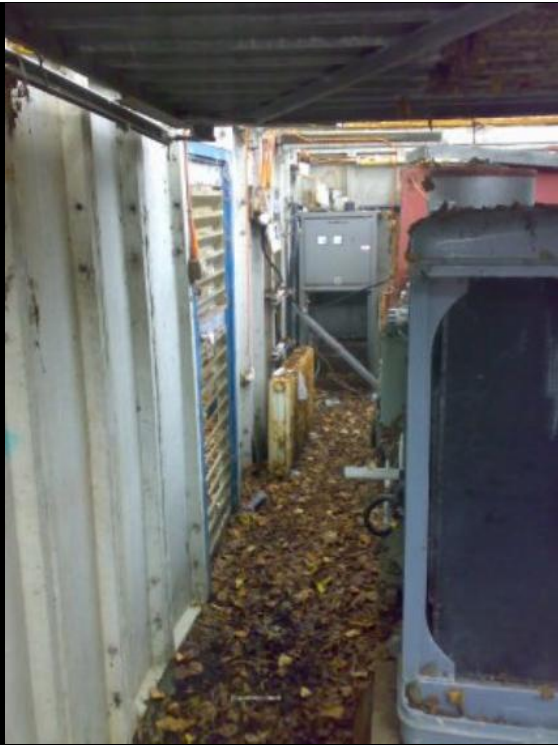
ABOVE: Switchgear next to the genny still appeared to be totally functional!
