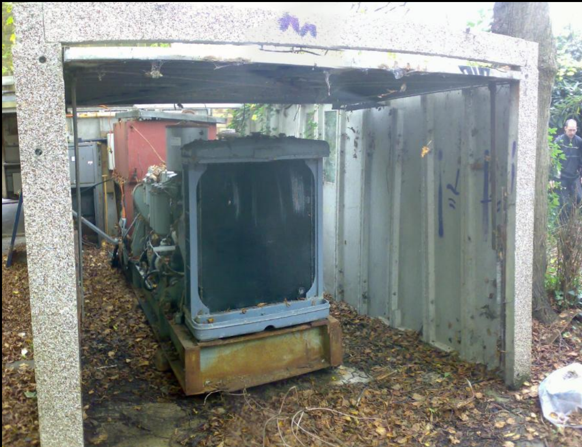
Ahhhh. You can't beat a good old fashioned BFG. Ever hospital should have one. ( A Big F***ing Generator). We did wonder if it would still work (quite possibly) but the entire planet would have heard it, methinks.
