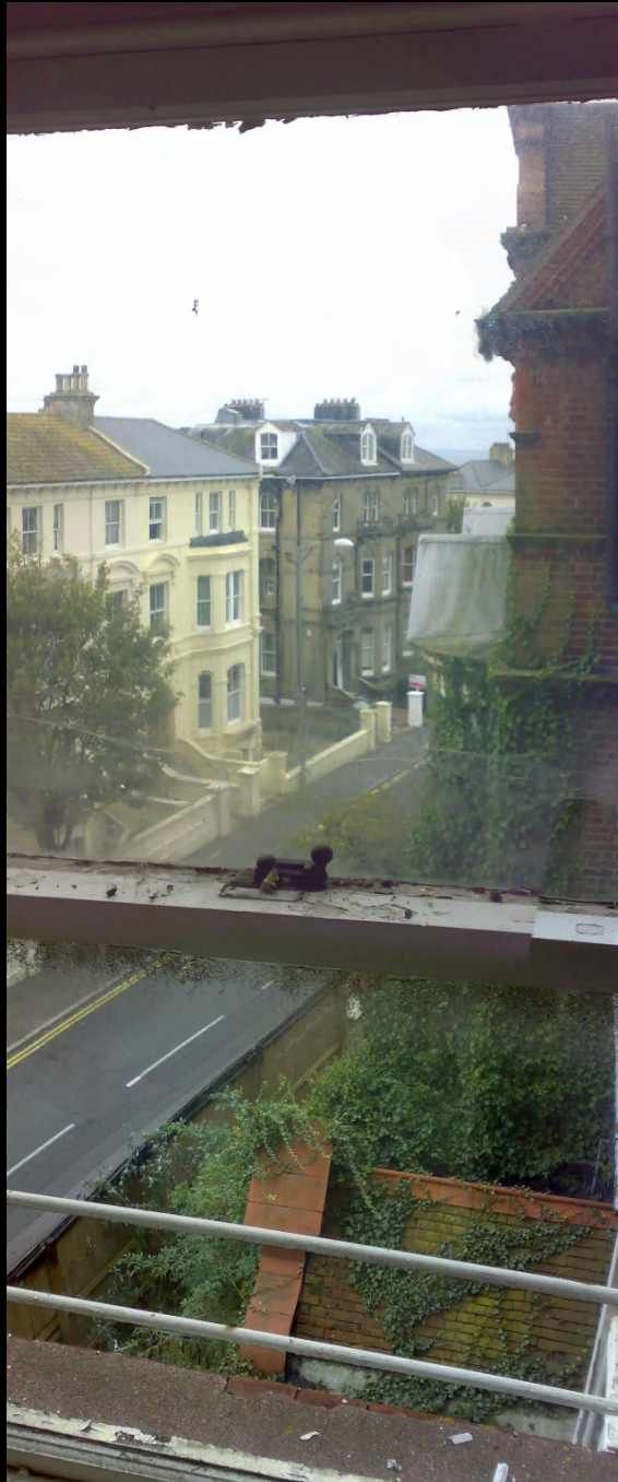
ABOVE: This is the view from the third floor immediately above the main entrance, looking due South towards the seafront. This picture shows some of the incredibly ornate brick and tile work on the exterior of the original building. Nature is taking a hold and is gradually reclaiming the Royal Alex Hospital.
