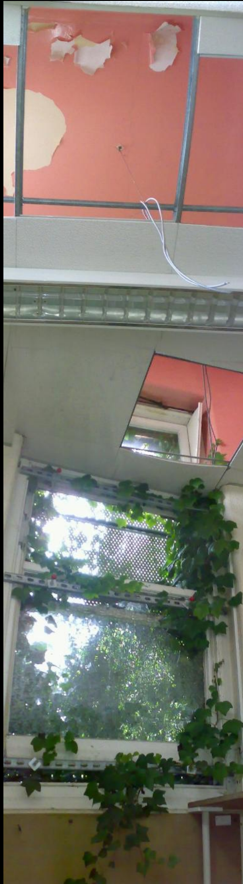
ABOVE: Okay, bit of a weird shot here, but I was trying to capture the way that the false ceilings had been put in with total disregard for the original window height. It's nice that the ivy was coming in both above and below the false ceiling. It would be interesting to come back in 3 months or so and see how the ivy has progressed.
