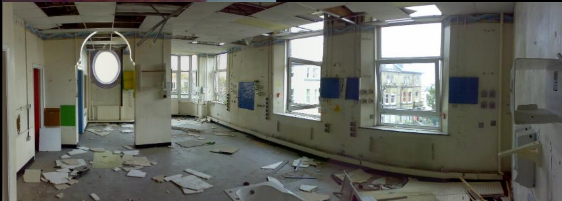
ABOVE: Open Ward inside the South-Eastern frontage. I wish I'd taken a shot of the oval window looking through the arch. Again, note the installation of the false ceiling with total disregard for the height of the windows. Looking through the gaps in the ceiling tiles unearthed some quite ornate original ceiling roses.
