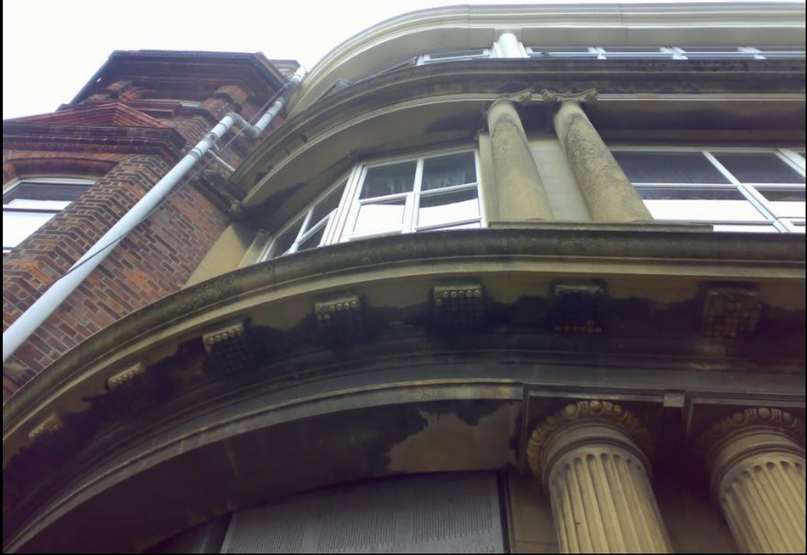
BELOW: Back to the south-west corner - retracing our steps incase we missed something. A well hidden way in, perhaps?
