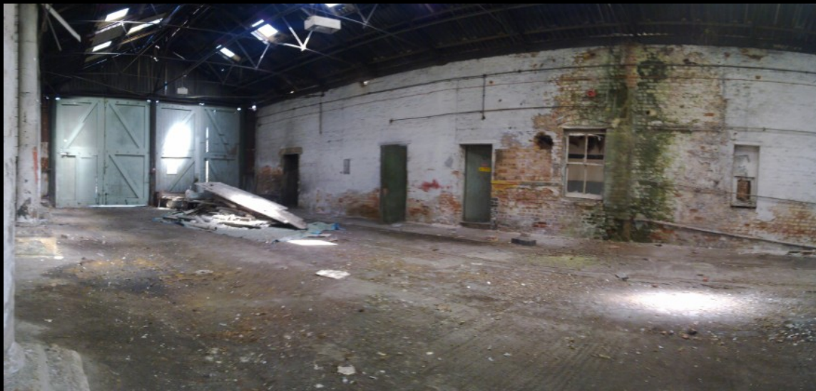
BELOW: The opposite view of the photo above, looking into the building from the left of the double doors seen in the last photo. The pillars are cast iron and date from 1882. Fantastic!
