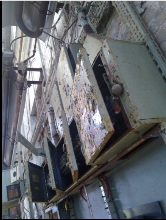
BELOW; This part of the site shows possibly the most recent changes to the site: this area looks like it has been set up as a spray booth for paint spraying. The nut&bolt and fixing stores can be seen in the background, centre of the photo.
