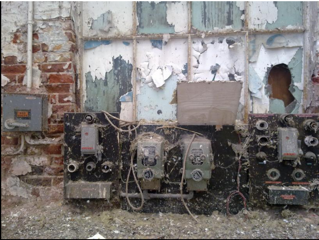
ABOVE & BELOW: Some of the switchgear in more detail. It was at this point that a pidgeon relieved itself all over Ghost...
