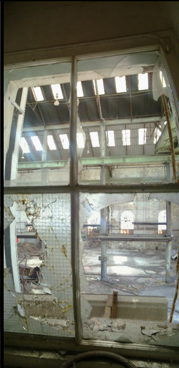
BELOW: External view of the main workshop building, showing those lovely windows.
