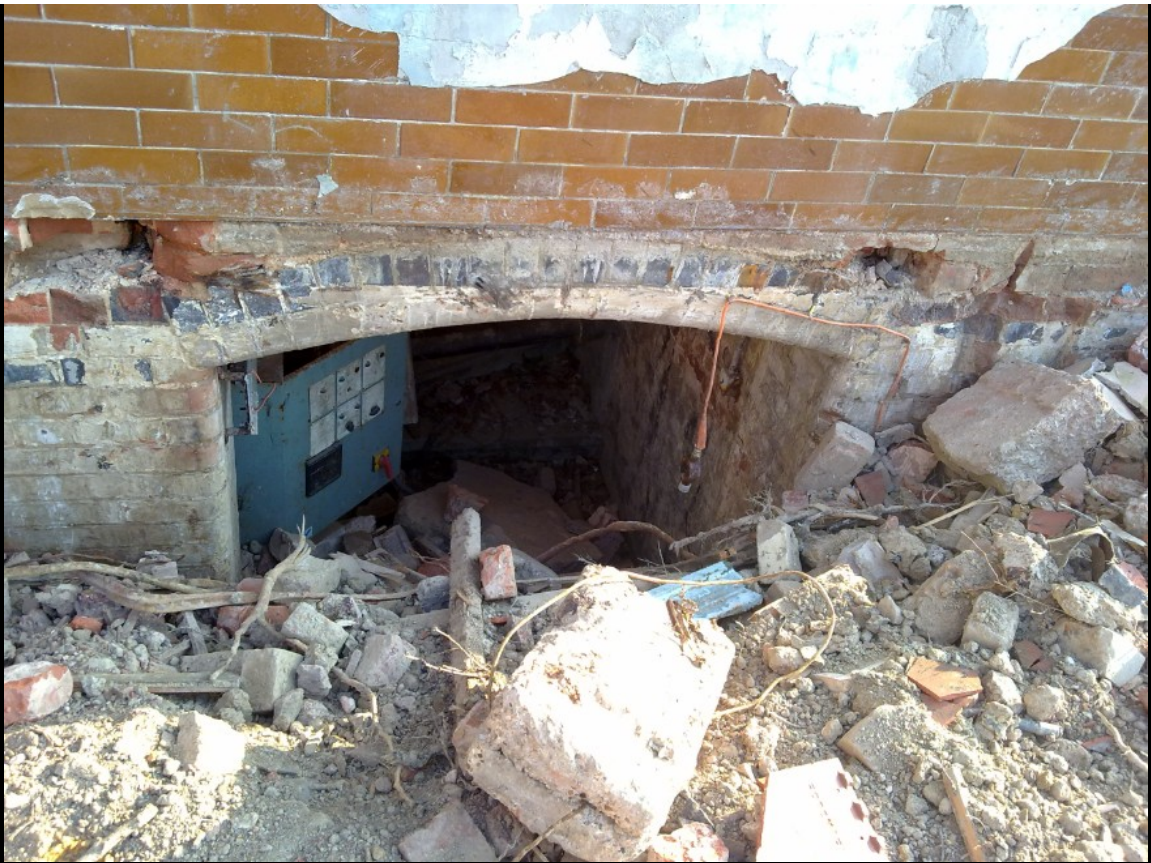
ABOVE & BELOW: The vast majority of Hellingly's enormous network of service tunnels was filled in between May and July 2010, but it's nice to see a few little bits of them still remaining defiantly. It was ever so tempting to get down into them and have a look, but would I have got out again?
