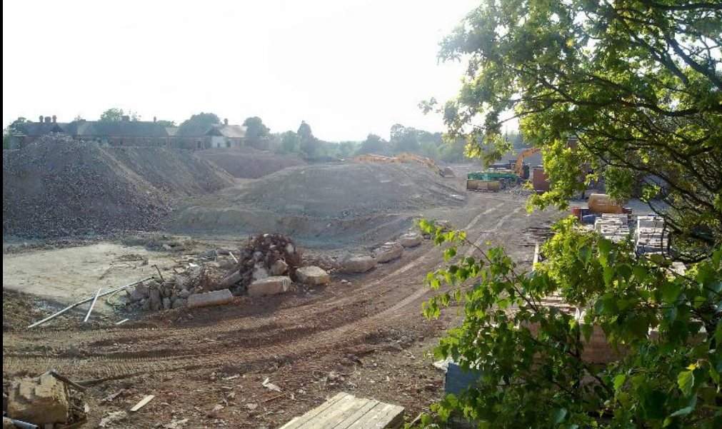
ABOVE & BELOW: This is the central nucleus of the site as it once was, looking from The Nurses' Accommodation Block. The Water Tower would have stood just where the excavator is, with the jib stretched out. The Main Hall would have been just to the left of this photo and the kitchens and laundry area would have been dead centre of the photo. A lot of the brickwork heaped up here is the remains of The Hall. It is hard to believe that the same view (from a couple of feet to the left) is seen in happier times, BELOW.
