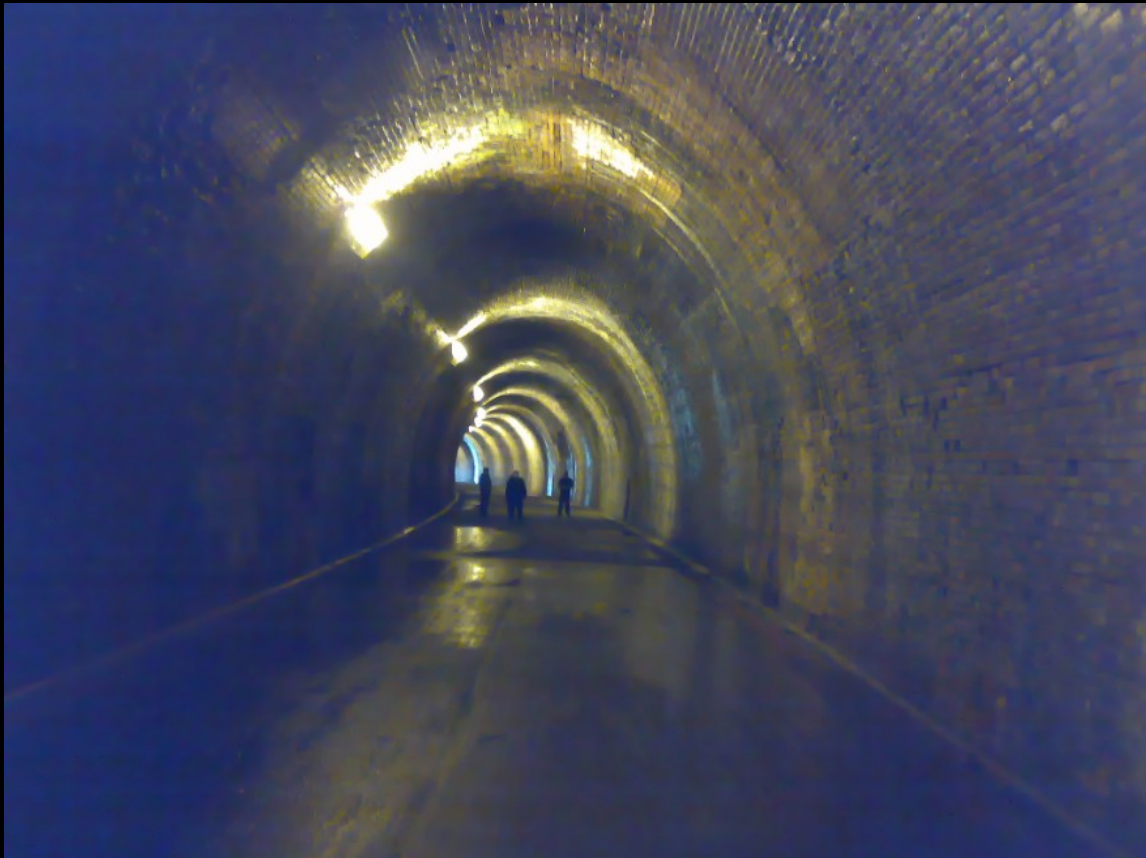
BELOW: The brickwork in the tunnel is in excellent condition and provides a fascinating collage of colour due to the varying combinations of fungi, soot and water ingress.
