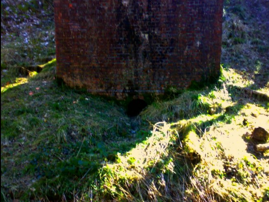
BELOW: An arty shot of one of the support piers from horizontal through to vertical. I love the range of colours caused by weathering, water ingress and soot over the course of just over a century (Nick? LOR).
