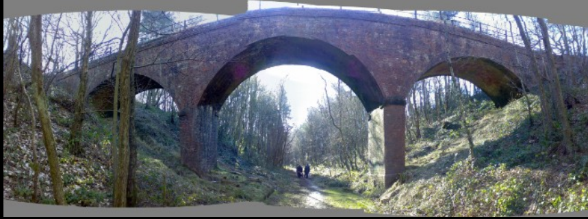
BELOW: Again, the brickwork is in excellent condition as can be seen from these photos of the support piers. Note the integral drainage duct built into the pier - this is quite an uncommon feature in bridges, but a very clever one.
