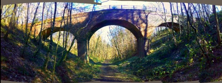
ABOVE: Panoramic view of the whole bridge. It is in excellent condition, with very little deterioration of brickwork at all. It also appears not to have been re-patched, which is incredible considering how long it has been here. NB: The curve of the bridge is artificial and caused by the 'indexing' of the camera from left to right.
