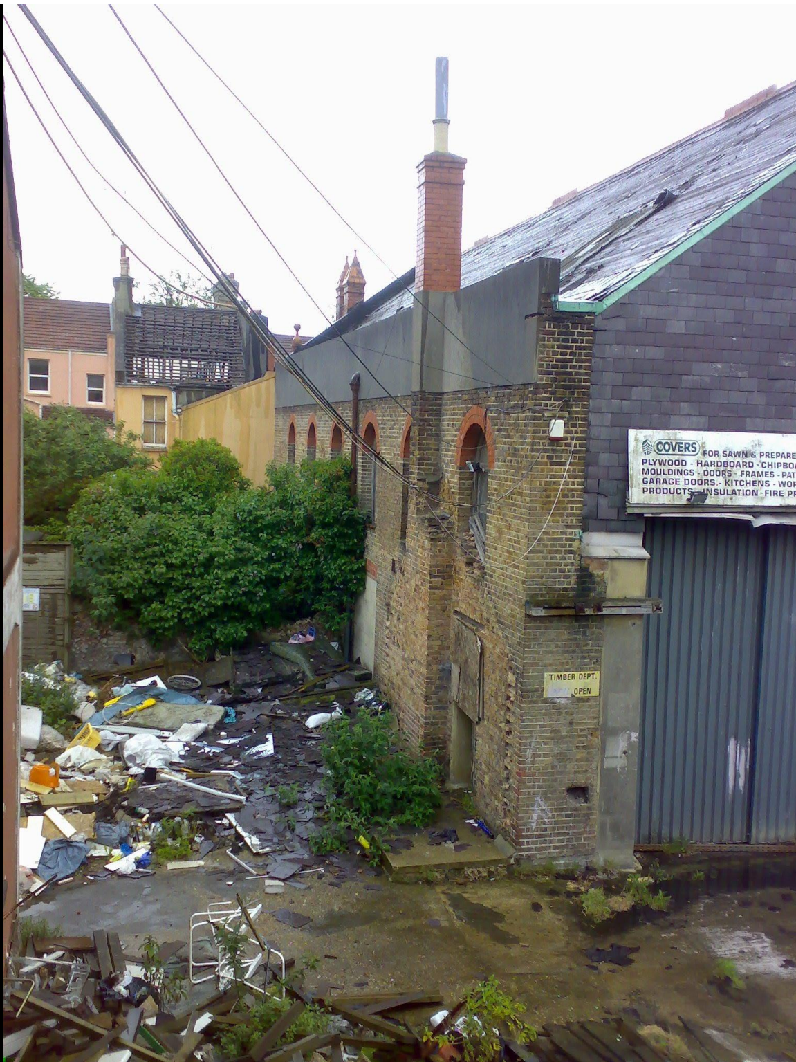
ABOVE: Close shot of our only possible way in. The little doorway behind the board has also been boarded up from the inside, but it is just possible to see into the hall. Unfortunately, there was a huge pile of crap behind the inner board, which was impossible to move very much. We did try and lever it out the way and prop it up or move it, using the huge abundance of timber around the place, but this was quite noisy and as the area is largely residential, we had to admit defeat on the main hall. We're thinking about going back on a week day and having another go. Watch this space....
