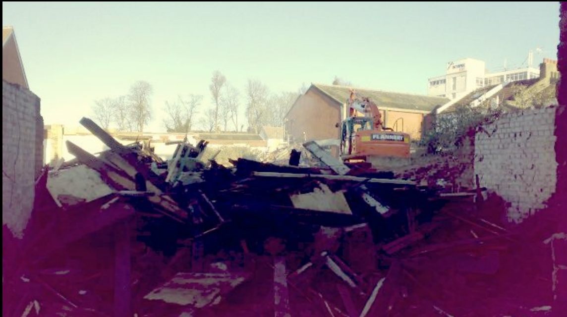
ABOVE: Connaught house has been razed to the ground and with the exception of the last 2/3 of the facade, is little more than a pile of rubble now. The building just beyond the excavator is the building where we sheltered from the rain on the first visit.
