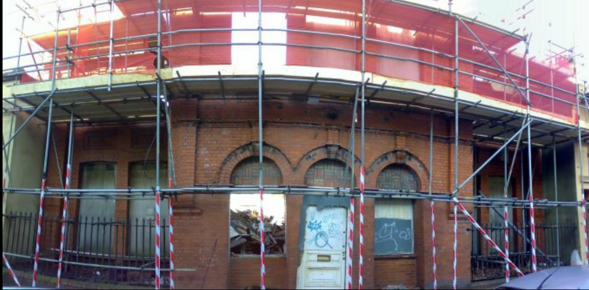
ABOVE: Going...going... The top third of the beautiful terracotta brick facade has gone! I will be back over the next couple of weeks as it comes down. The building beyond has vanished, as is evident from the pile of rubble visible through the window.
