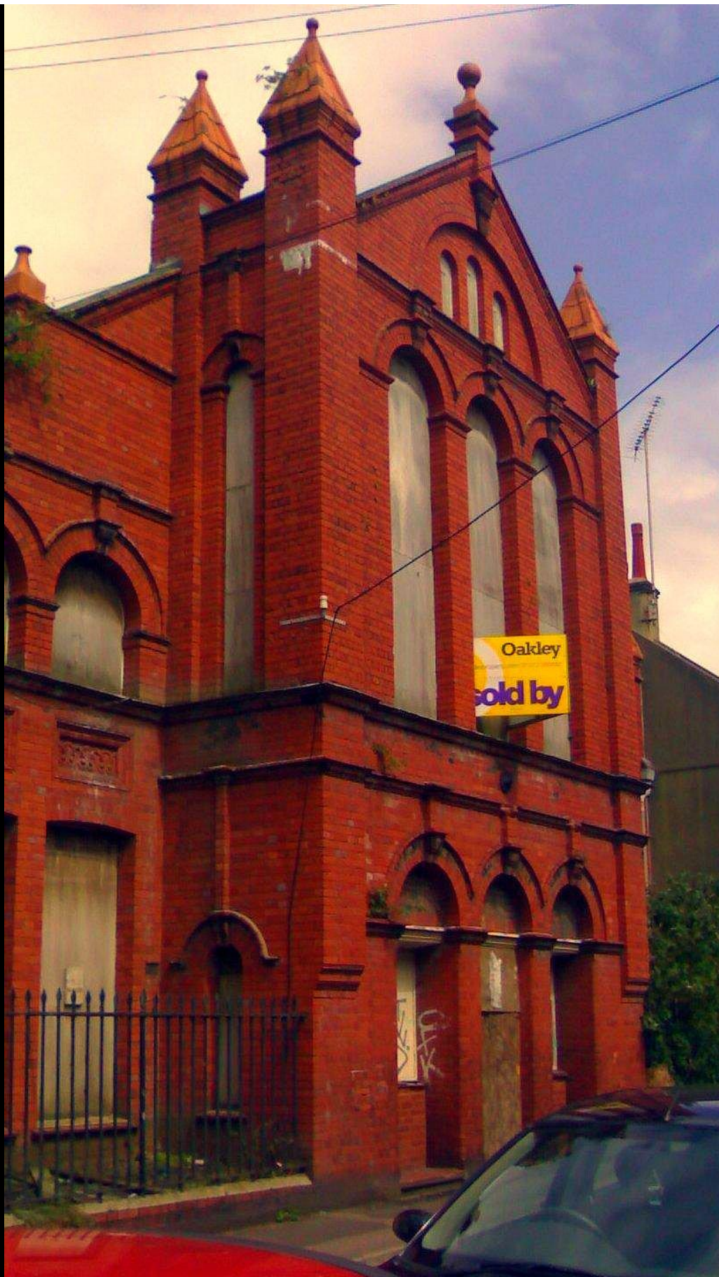
ABOVE: This is the fabulous terracotta frontage of Connaught House. Behind the railings there is a layer of plywood on the floor that doesn't look quite right. We had a closer look and through a gap in said wood, we found a 30foot deep drop to what appears to be a cellar level. There is a doorway boarded up down there and we are guessing that there must also be a flight of stairs leading down to it around the frontage somewhere. Despite the flimsy boards, which could be removed by any intending investigators in minutes, this end of the site is a highly residential area and is overlooked directly from the main Lewes Road, a horribly busy thoroughfare. Maybe if we have better luck on a return visit, we could get to the bit downstairs.
