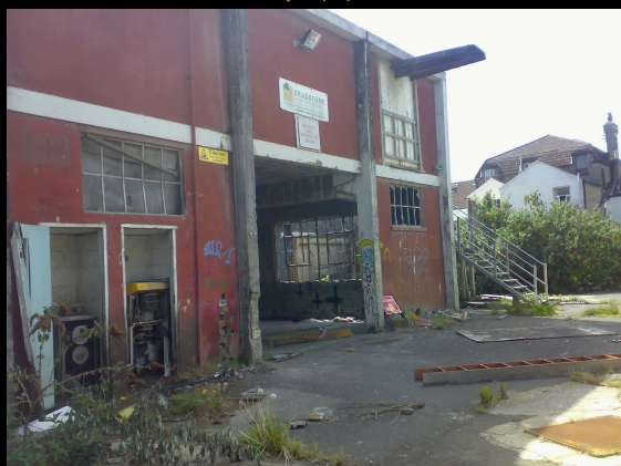
Above: access to the rear of the site looking roughly south-west. The main hall is just behind the flight of stairs.
